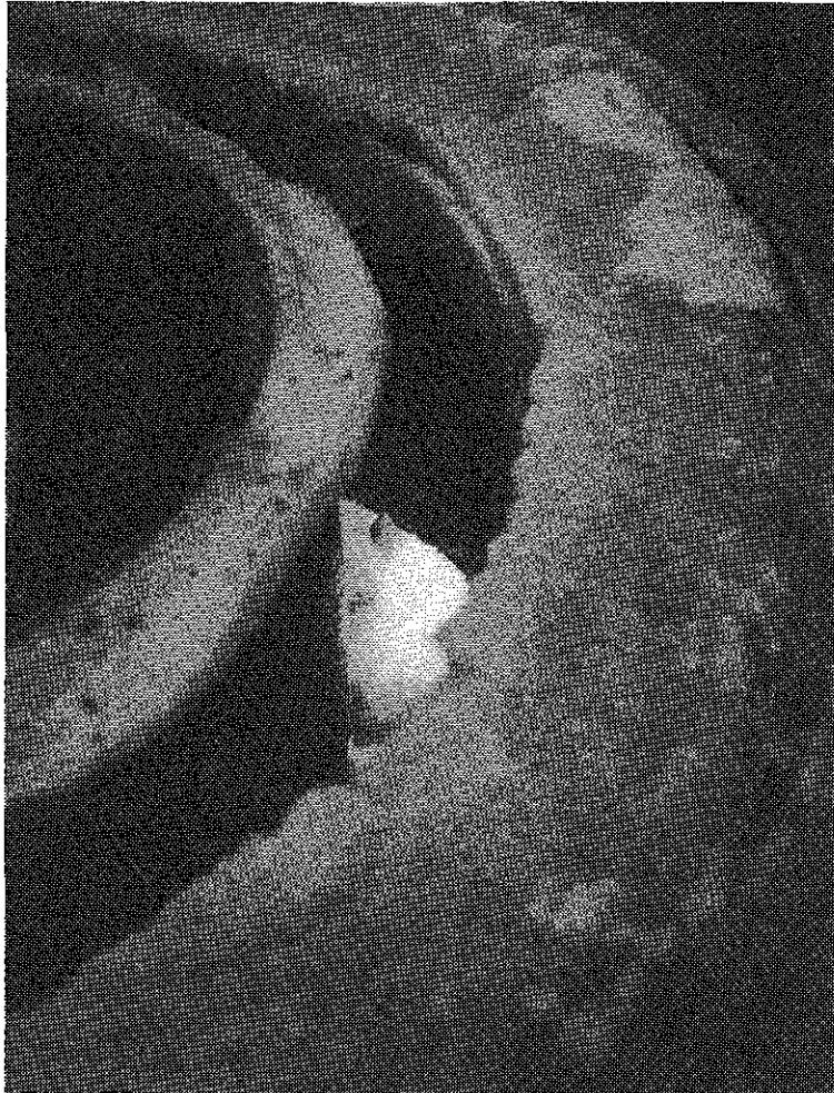
Figur 2.7 Brännare under drift
