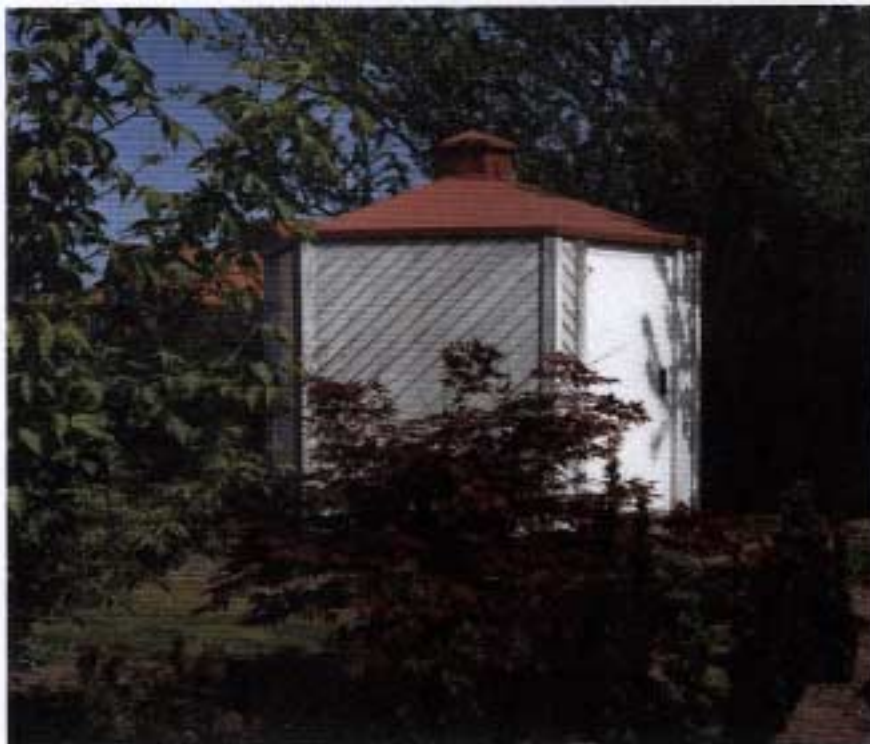
Figure 10 Regulating station in the Tivolitorget in Laholm, 10 MW connecting power
