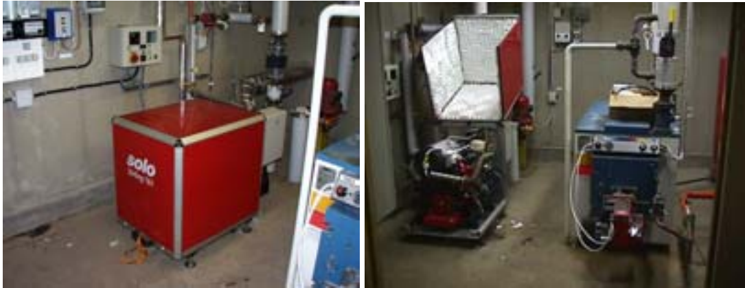
Stirling engine CHP-unit installed at the site in Gothenburg. Note exhaust pipe (aluminium coated) going through the wall and gas fired boiler (blue)
