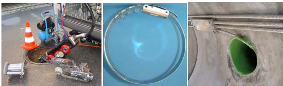
Figur 21. Installationsrobot FAST, (Fast Opticom, n.d.)
