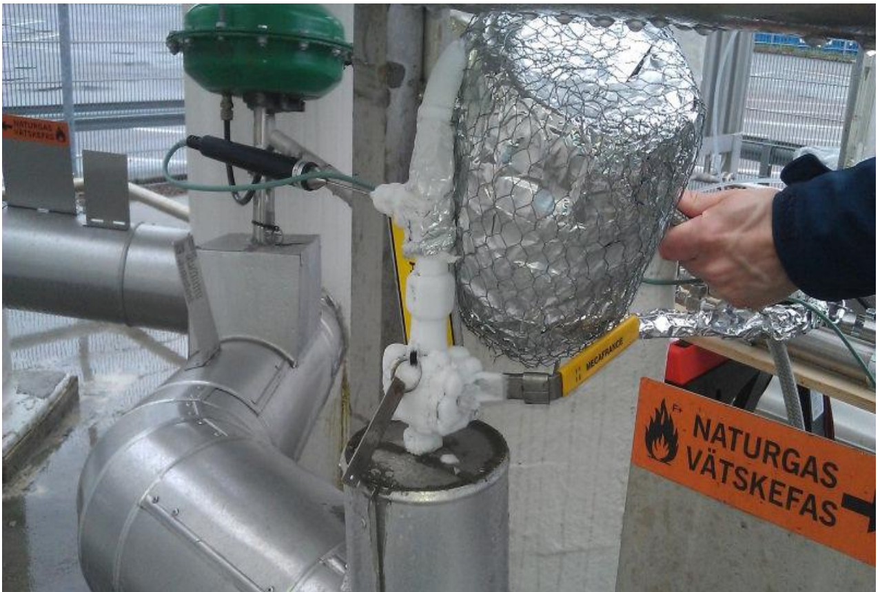
Figure 2.6: Picture of vaporizer connected to V66
